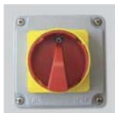
Electrical isolator fitted to fan for security
